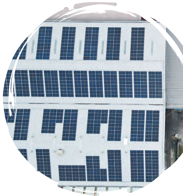
Solar panels have been installed at one of CBB's manufacturing facility in Senai, Johor
