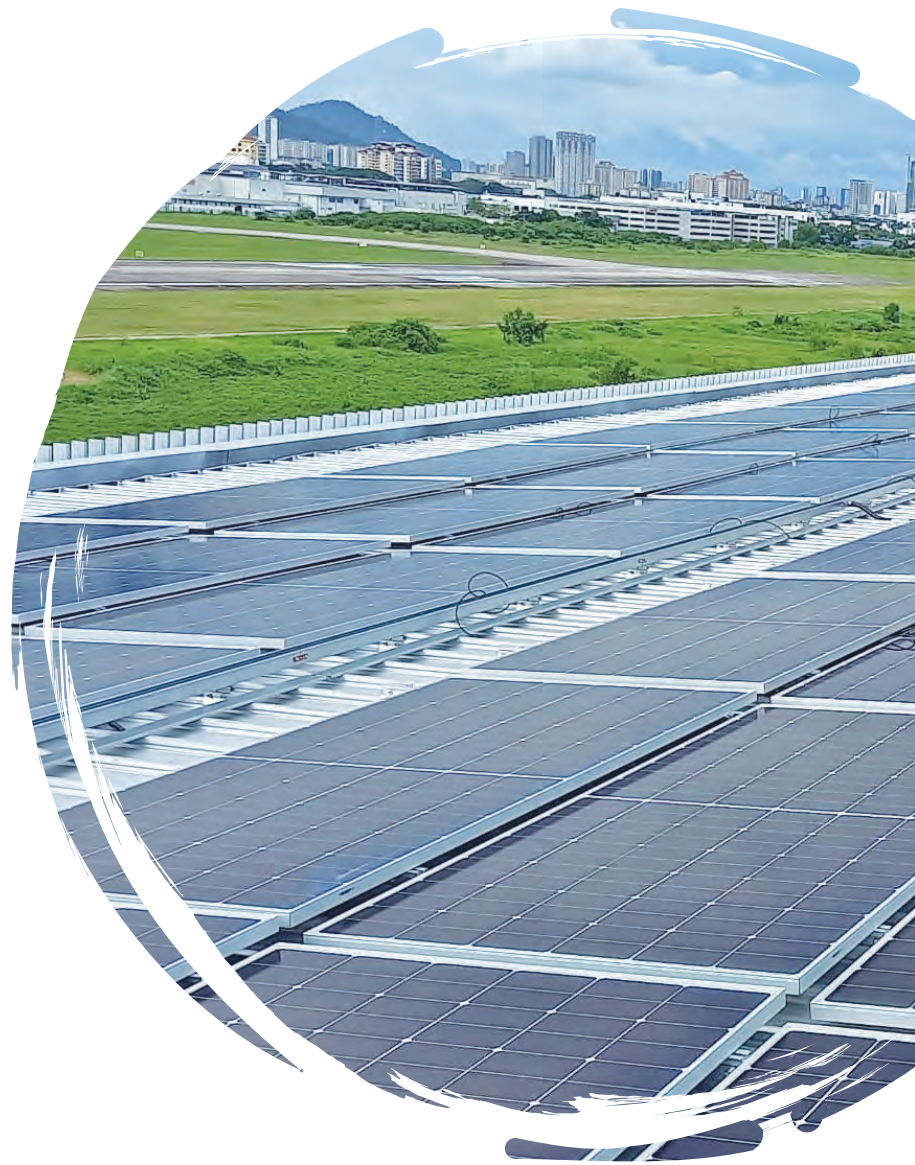
Harnessing the power of the sun: solar panels installation at CPI (Penang) Sdn. Bhd.
